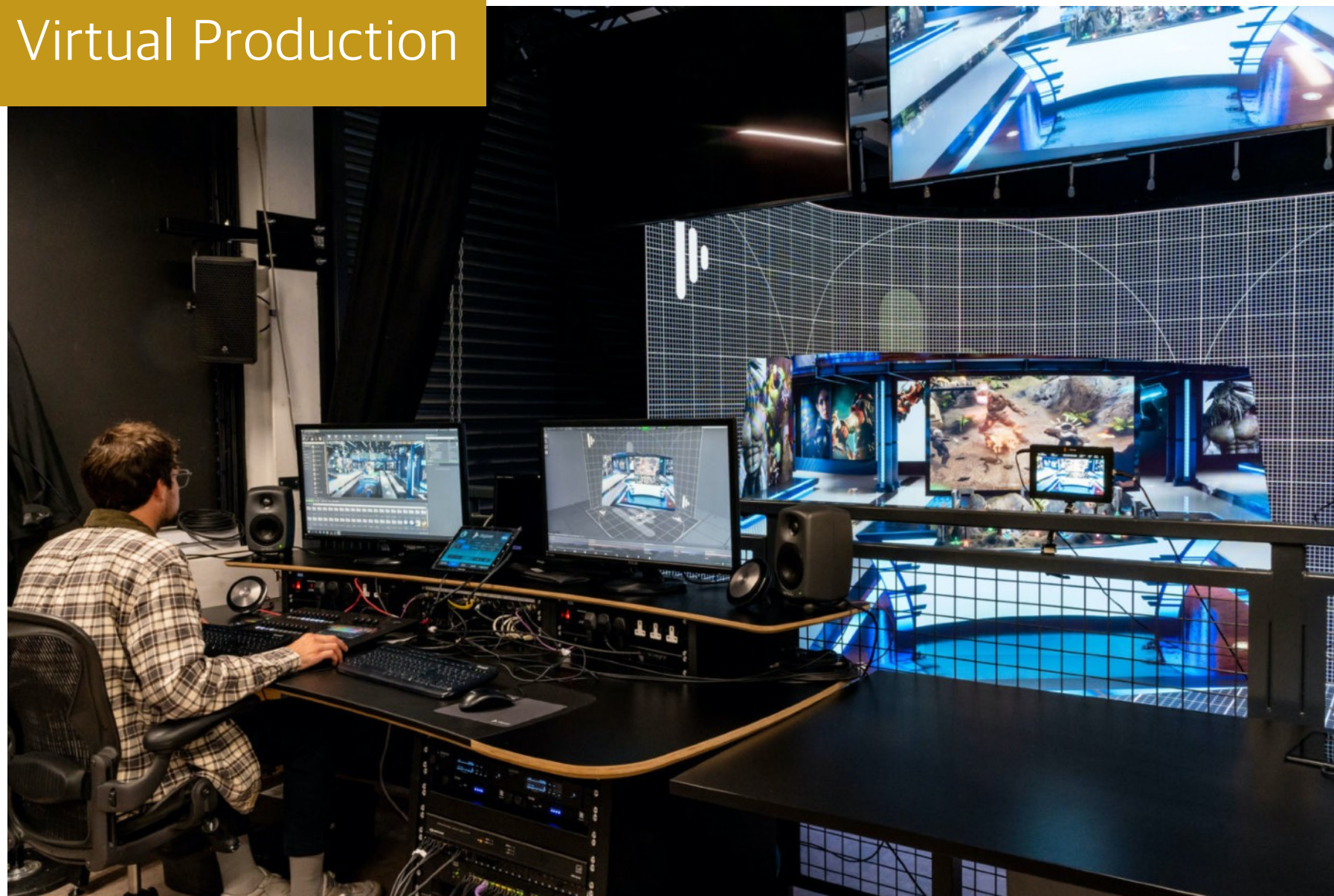
GPU Data Center
